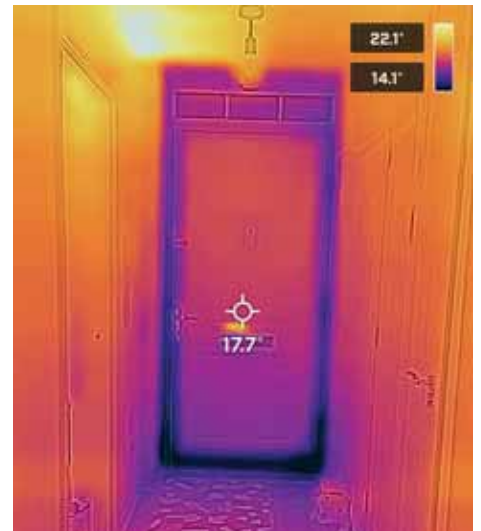
SWaCS member, Dave Smith took this thermal image inside the front door of his house built in 2018. It highlights the cold spots where heat is being lost that renewed insulating tape could cure.
